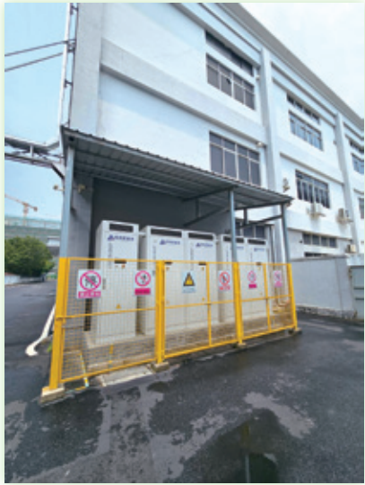
Figure 14. Battery Energy Storage Systems
